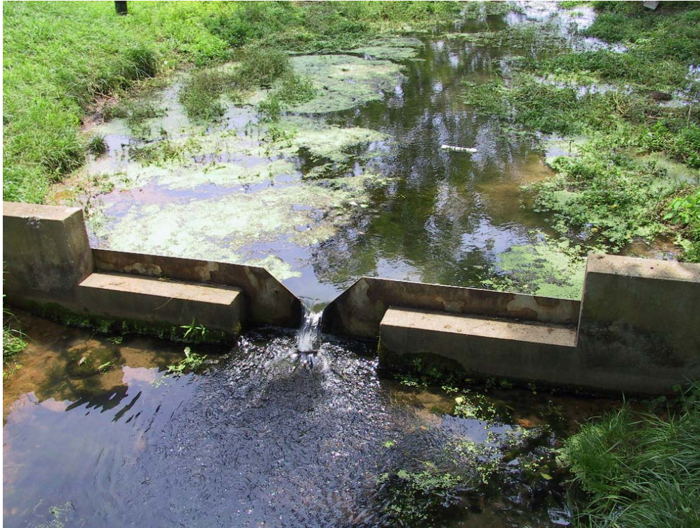
V notch weir in streamflow
